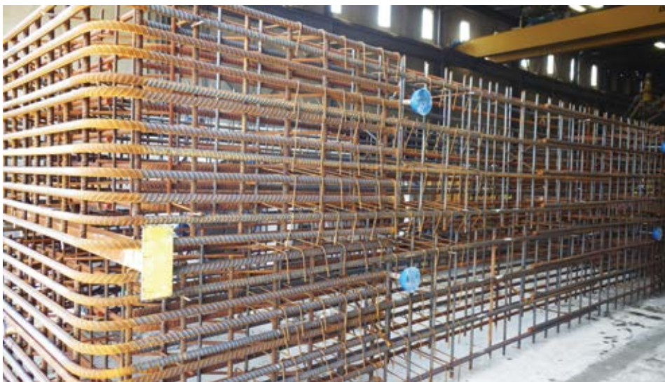
Rebar cages delivered from StelCrete, two cages per delivery, one stacked upon the other
