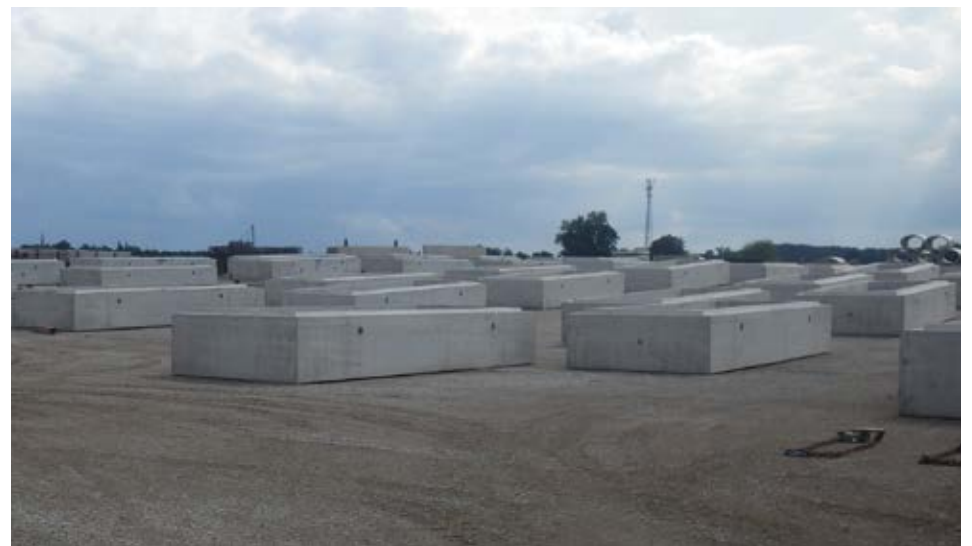
8000mm x 2100mm x 1.205m precast concrete sections ready for construction of M56 culvert
