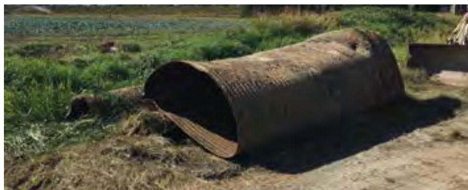
Severely corroded corrugated steel pipe Photos: The Langley Concrete Group of Companies
