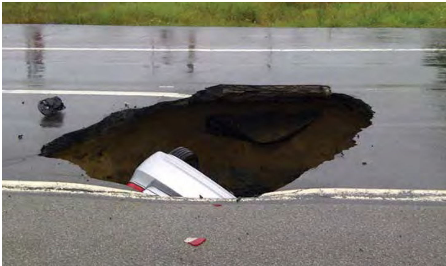
Car in hole caused by the collapse of a corrugated steel pipe – Highway 174, Ottawa, 2012
