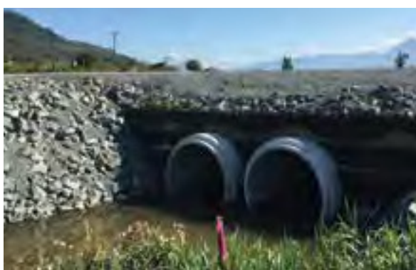
Concrete pipe, with a service life of more than 100 years, is now used for Chilliwack's critical infrastructure
