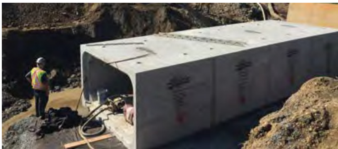
Chilliwack began specifying concrete pipe and precast concrete box culverts in 2015
